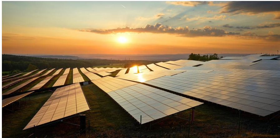
Photo:1 Solar Energy Panels
